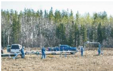
A work crew prepares to test a new brackish well and pipeline connected to Canadian Natural's Wolf Lake Central Processing Facility.
