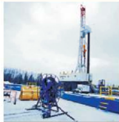
Imperial purchased the Alta 32E rig, which incorporates state-of-the-art features to keep people out of harm's way.
