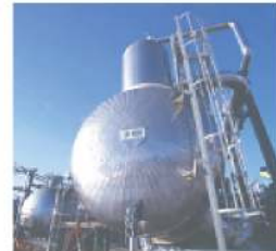
Cogeneration allows for otherwise wasted heat to power the entire Cold Lake operation while returning enough energy to Alberta's grid to power 50,000 homes.
