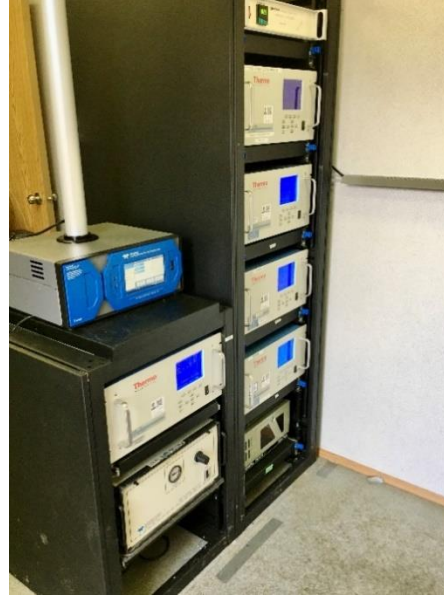
Interior (Instrument Rack)
